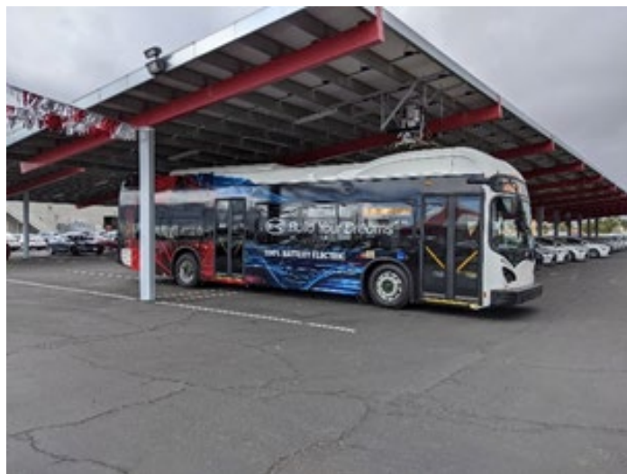
Figure 6. In-Depot Overhead Charging Example (Source: CALSTART)
