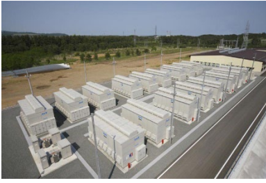
NGK NAS Battery System
