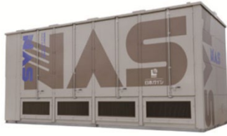
NGK NAS Battery Package Type Unit
